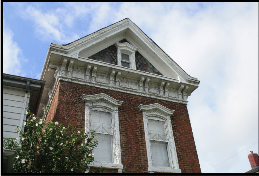
Photo 4 – Looking S at the second story of the front elevation of 905 Heaton street. Note the cornice work. Photo taken from Heaton Street.
